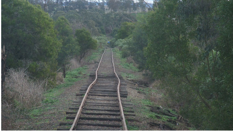
Figure 1. Photograph Showing Thermally Induced Buckling of a Railway (Reprinted with Permission from Lankyriders, CC BY-SA 4.0, via Wikimedia Commons)
