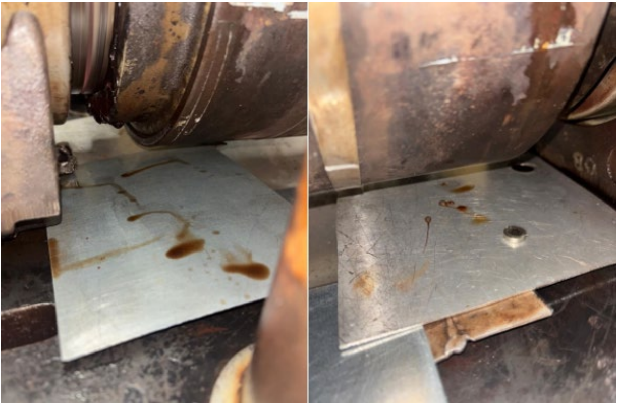
Figure 40: Leaked grease accumulation on IB (L2) and OB (R2) sides (12/31/2024)
