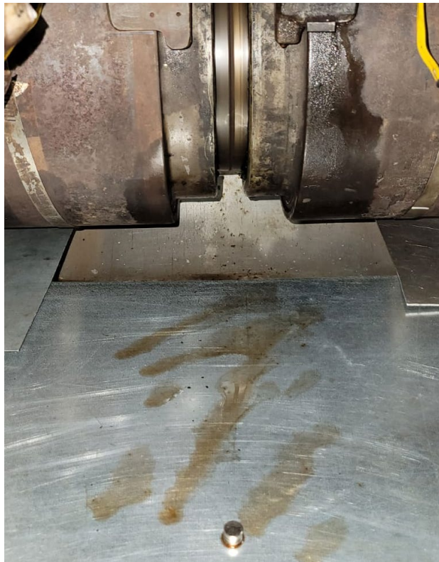
Figure 38: Leaked grease accumulation on OB (L2) and IB (R2) sides (12/27/2024)
