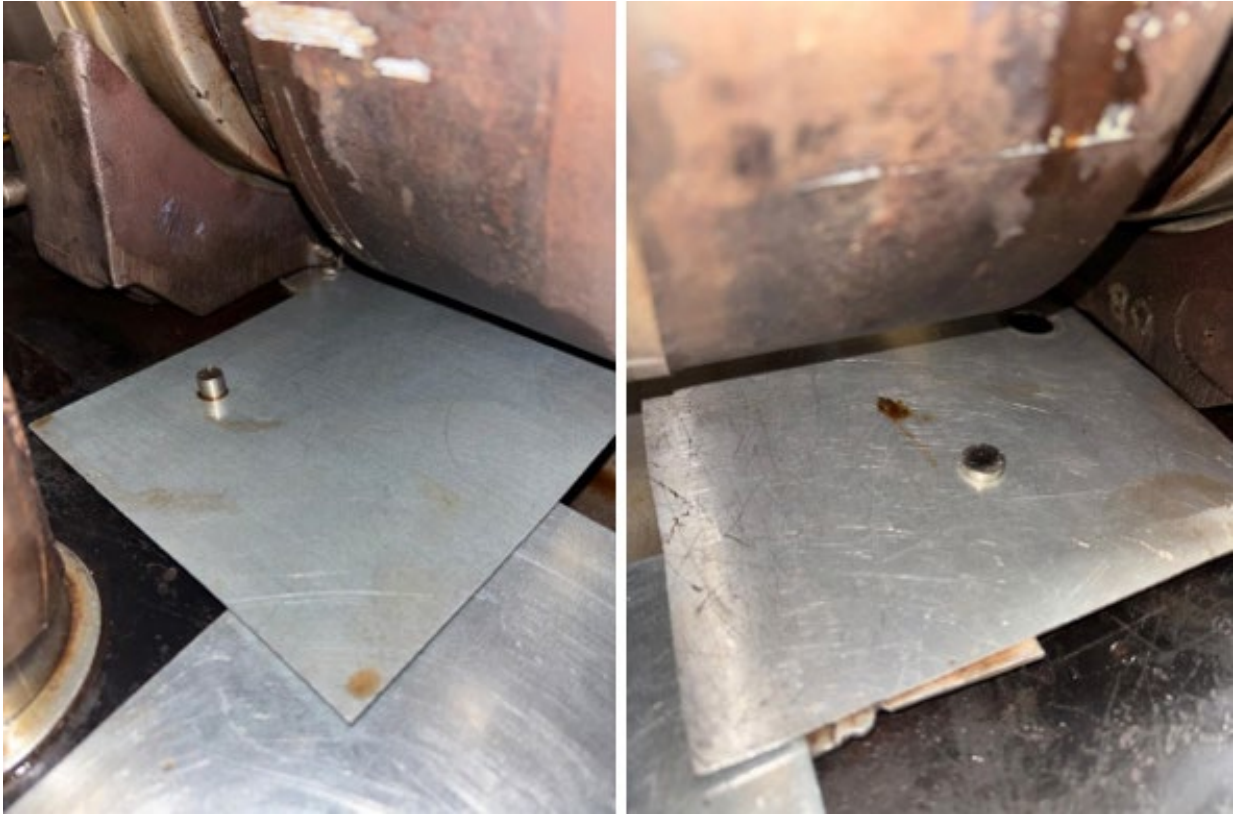
Figure 42: Leaked grease accumulation on IB (L2) and OB (R2) sides (01/08/2025)
