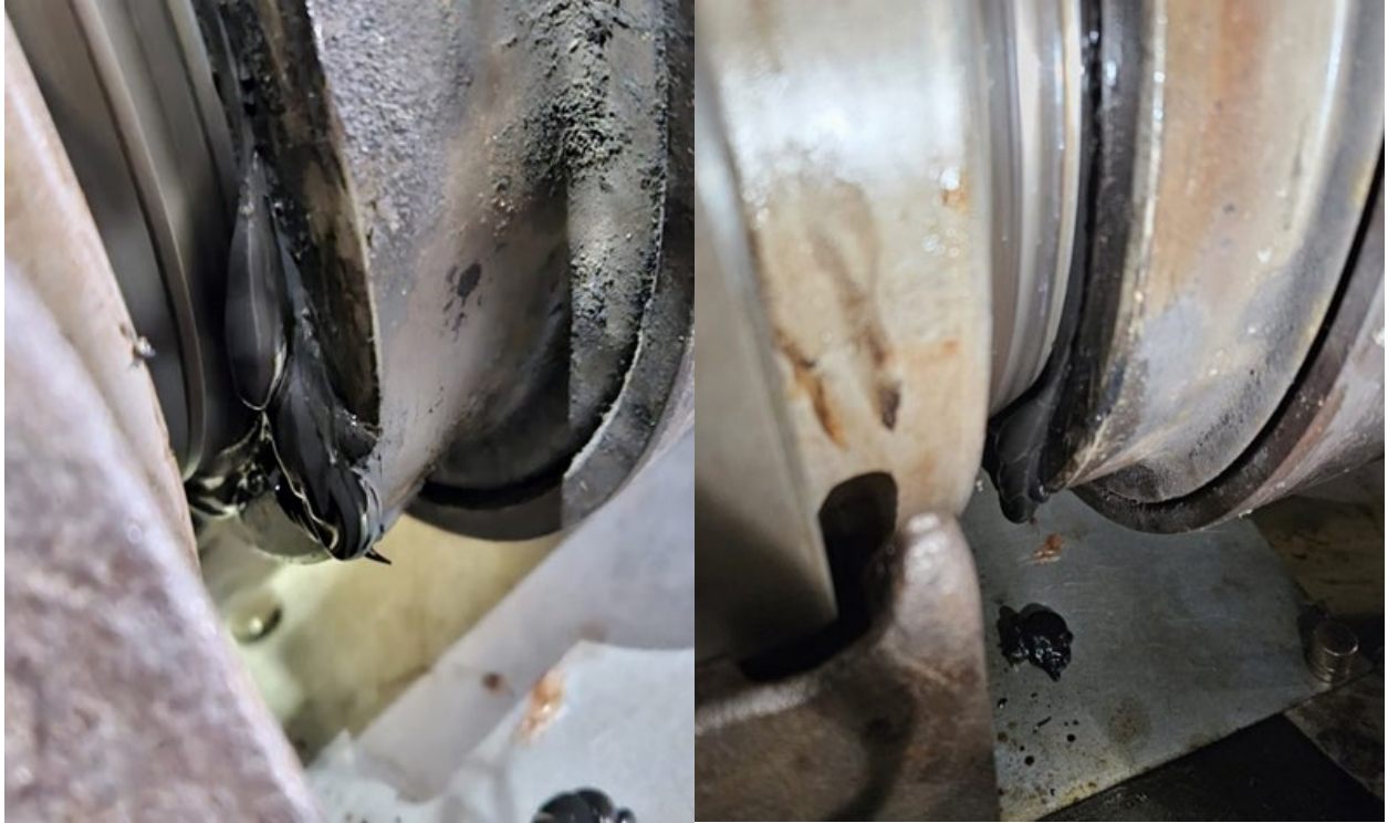
Figure 31: Grease leaking from the IB seal of Bearing L2 (11/05/2024)
