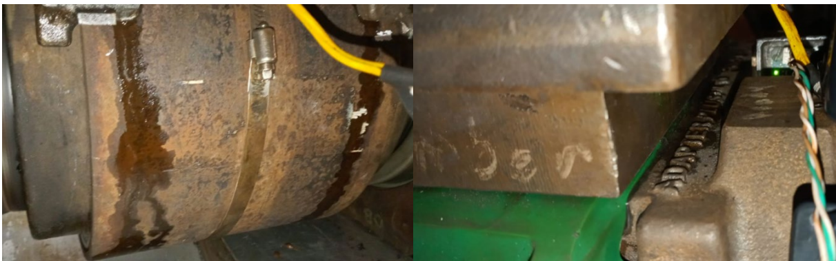
Figure 9: Pictures showing grease leak from bearing R4
