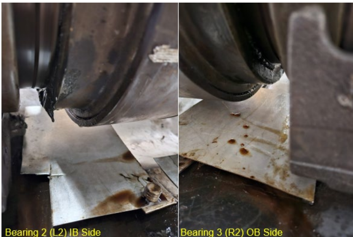
Figure 34: Leaked grease accumulation on IB (L2) and OB (R2) sides (11/14/2024)
