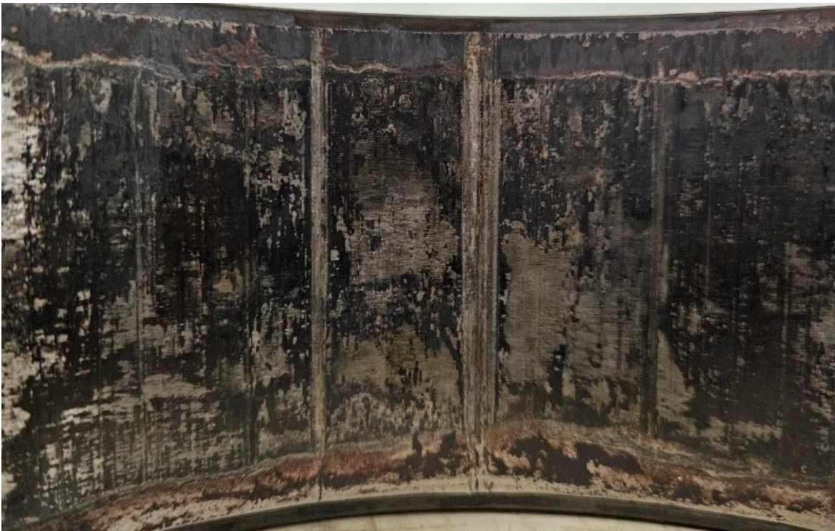
Figure 13: R4 IB cone inner diameter surface
