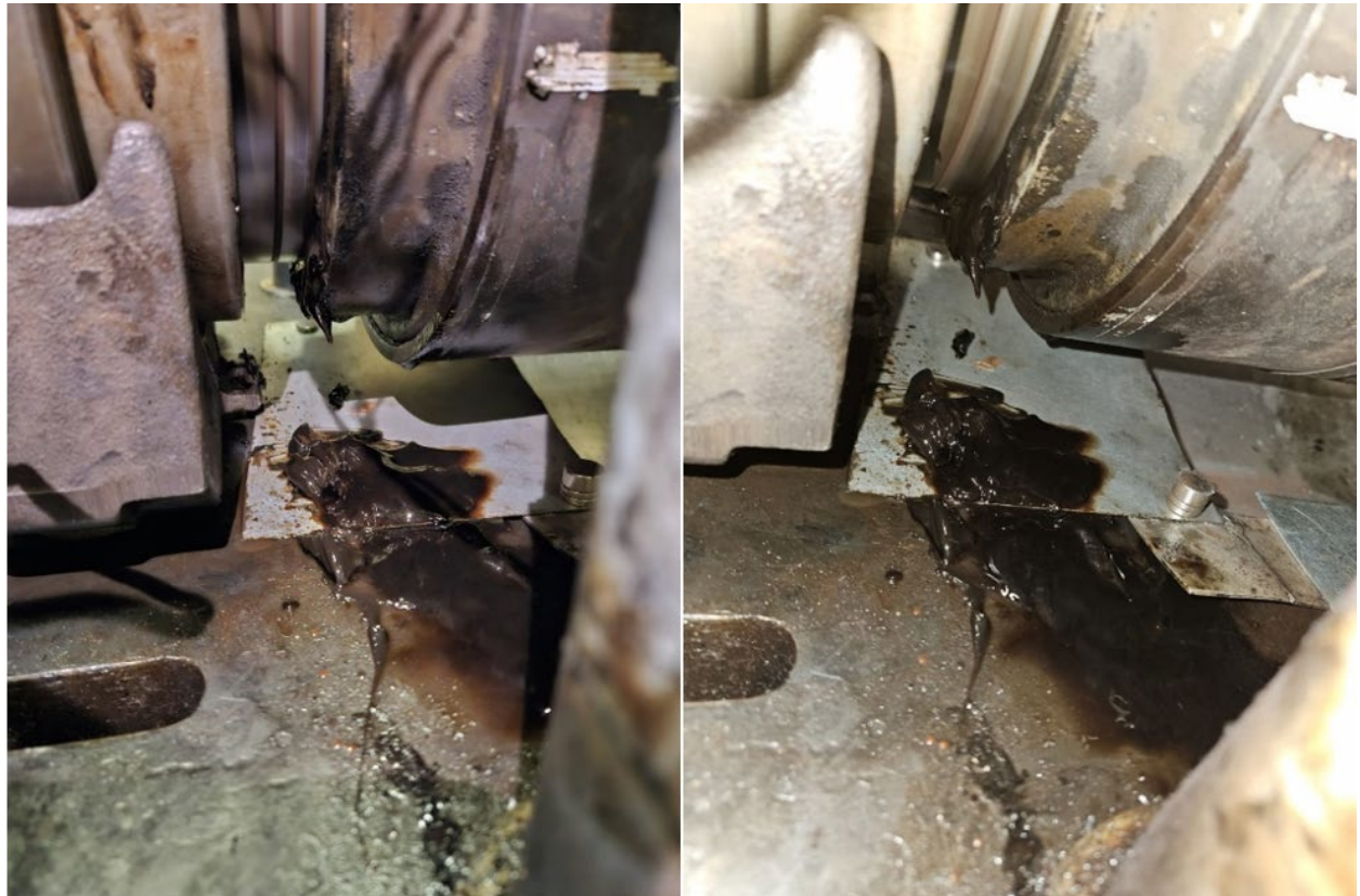
Figure 32: Leaked grease accumulation on IB side of Bearing L2 (11/08/2024)
