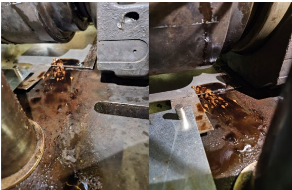
Figure 33: Grease leaking from OB seal of Bearing R2 (11/11/2024)
