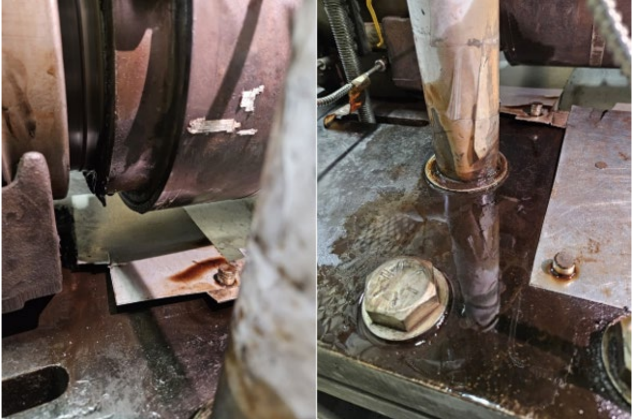
Figure 35: Leaked grease accumulation on IB side of Bearing L2 (11/18/2024)
