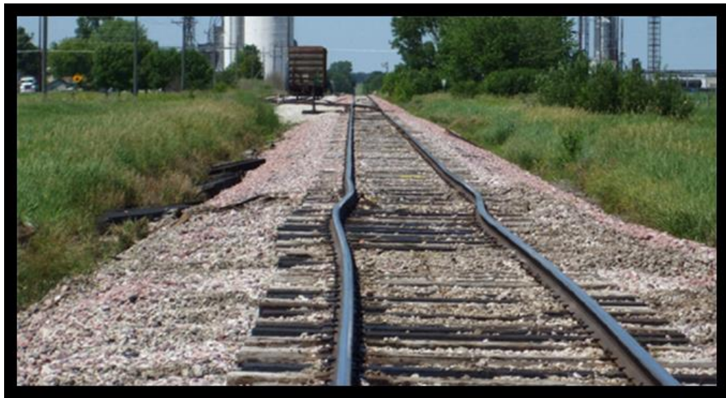
Fig. 8 Photograph Showing Thermally Induced Buckling of a Railway
