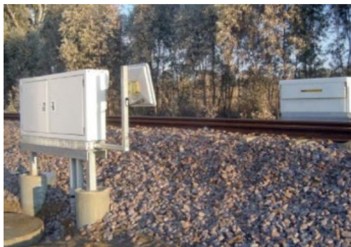
Figure 7. RailBAM (Rail Bearing Acoustic Monitor) site [16]
