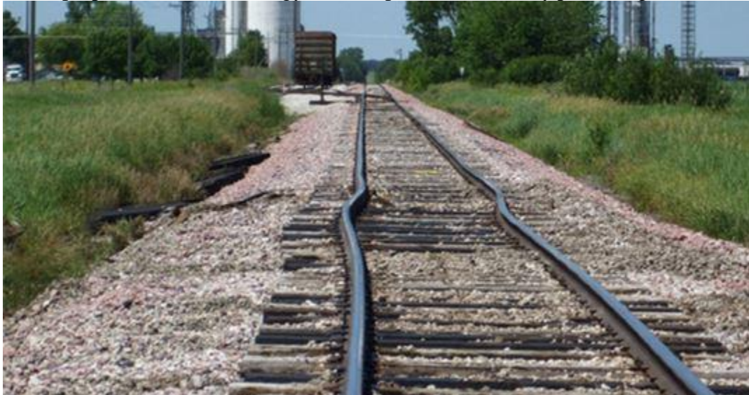
Fig. 1 Photograph Showing a Local Railway Buckle
