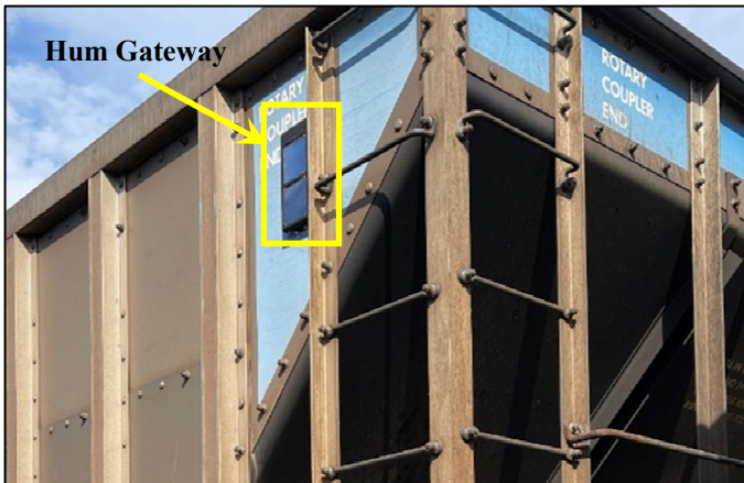
FIGURE 1: HUM GATEWAY INSTALLATION
