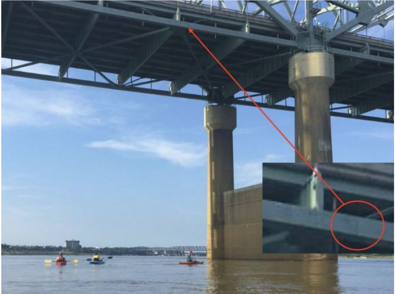
Figure 1: Bridge crack illustrating structural degradation - [9]
