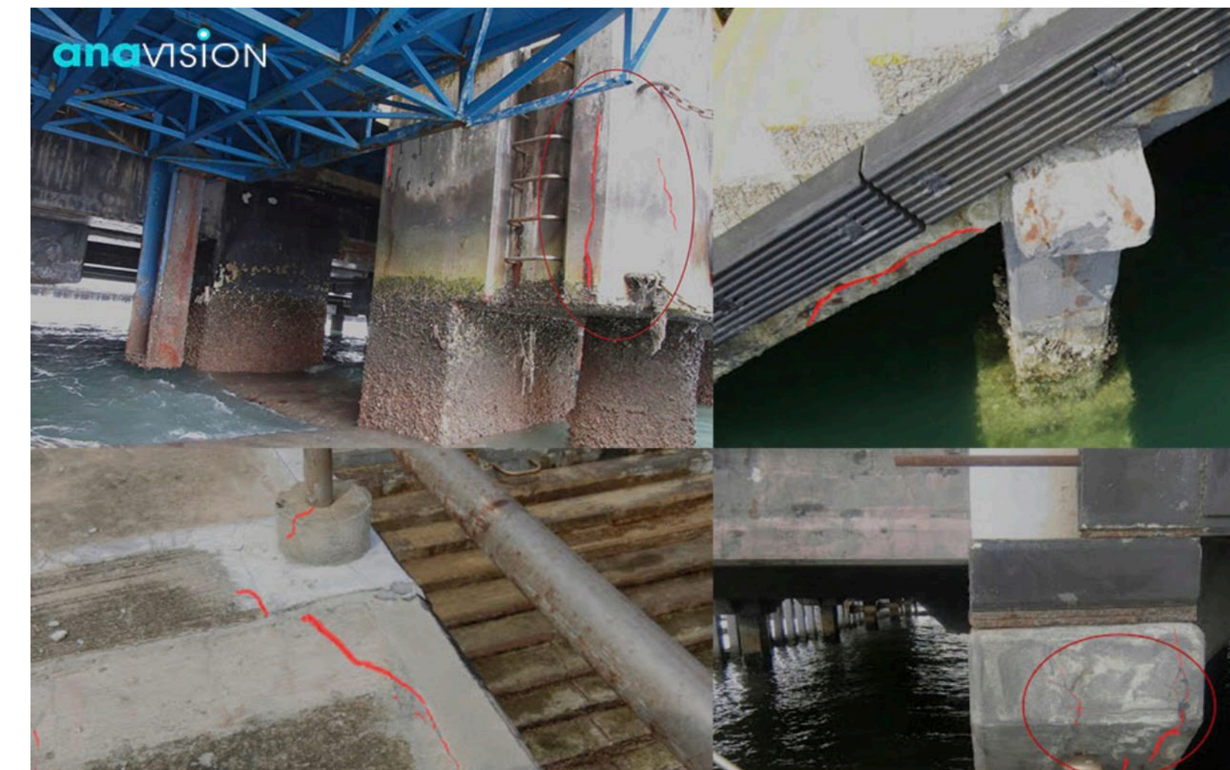
Artificial Intelligence Pier Crack Detection [6]
